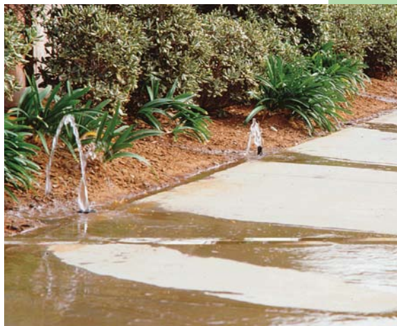
Run-off and wasted water when check valves are not installed.
