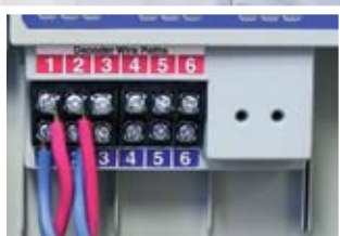
Two-wire Decoder Control of up to 99 Stations
