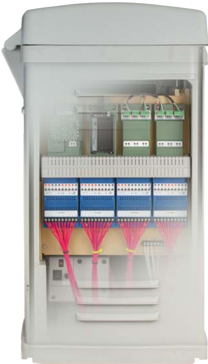
Pilot Field Controllers: Conventional solenoid wiring with an individual wire running to each valve.
