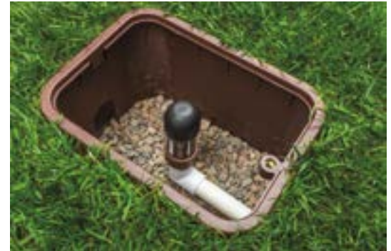
Air/Vacuum Relief Valve Installed
