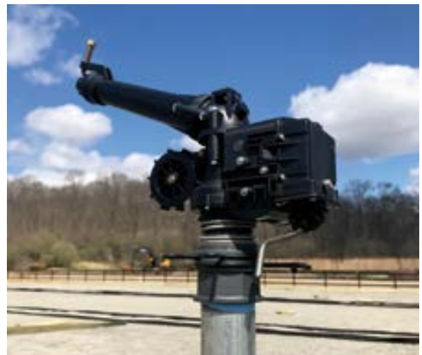
ST-1200-BR Rotor Installed
