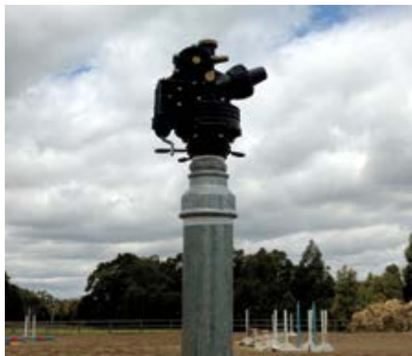
ST-1600-HS-BR Rotor Installed
