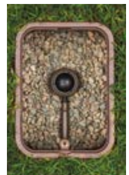
Automatic Flush Valve Installed
